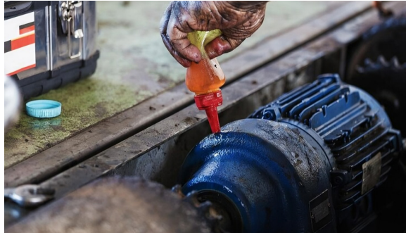
Fig. 3.5.3: Lubricating Moving Parts for Smooth Operation
